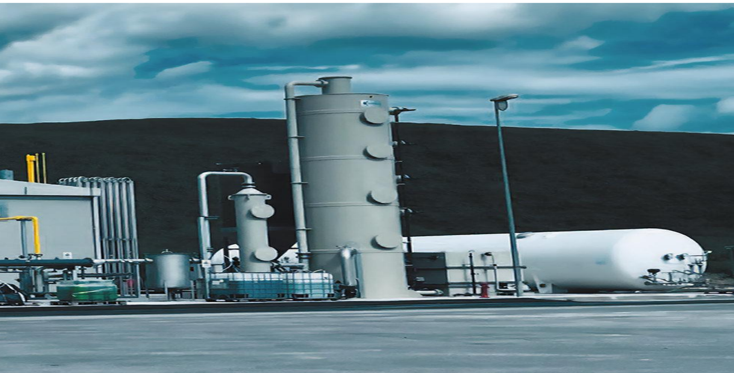
Liquefied CO 2 Cylinder at coal-fuelled power station that can be transported to suitable CO 2 sequestration site
